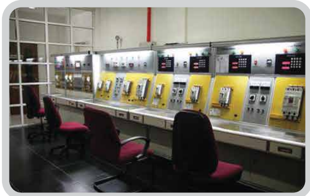
GENERAL VIEW OF MCB AND MCCB TESTERS
