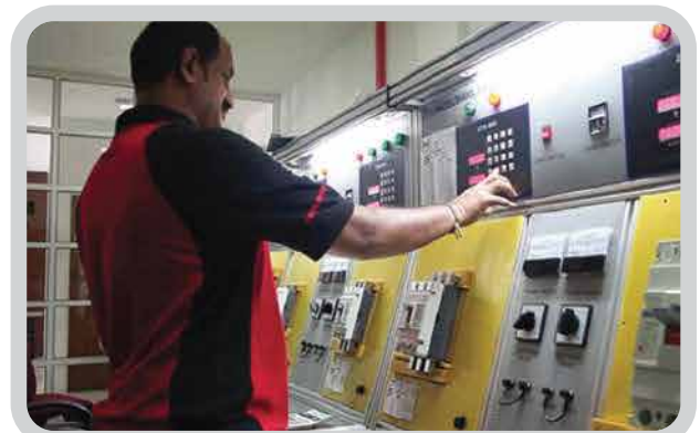
MCCB OVERLOAD CALIBRATION TESTER
